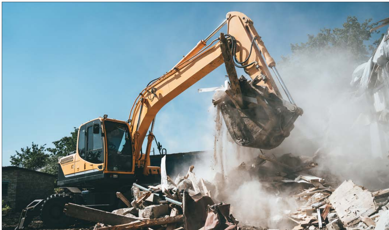
The cost of demolition also depends on how much of the demolition material can be recycled.
